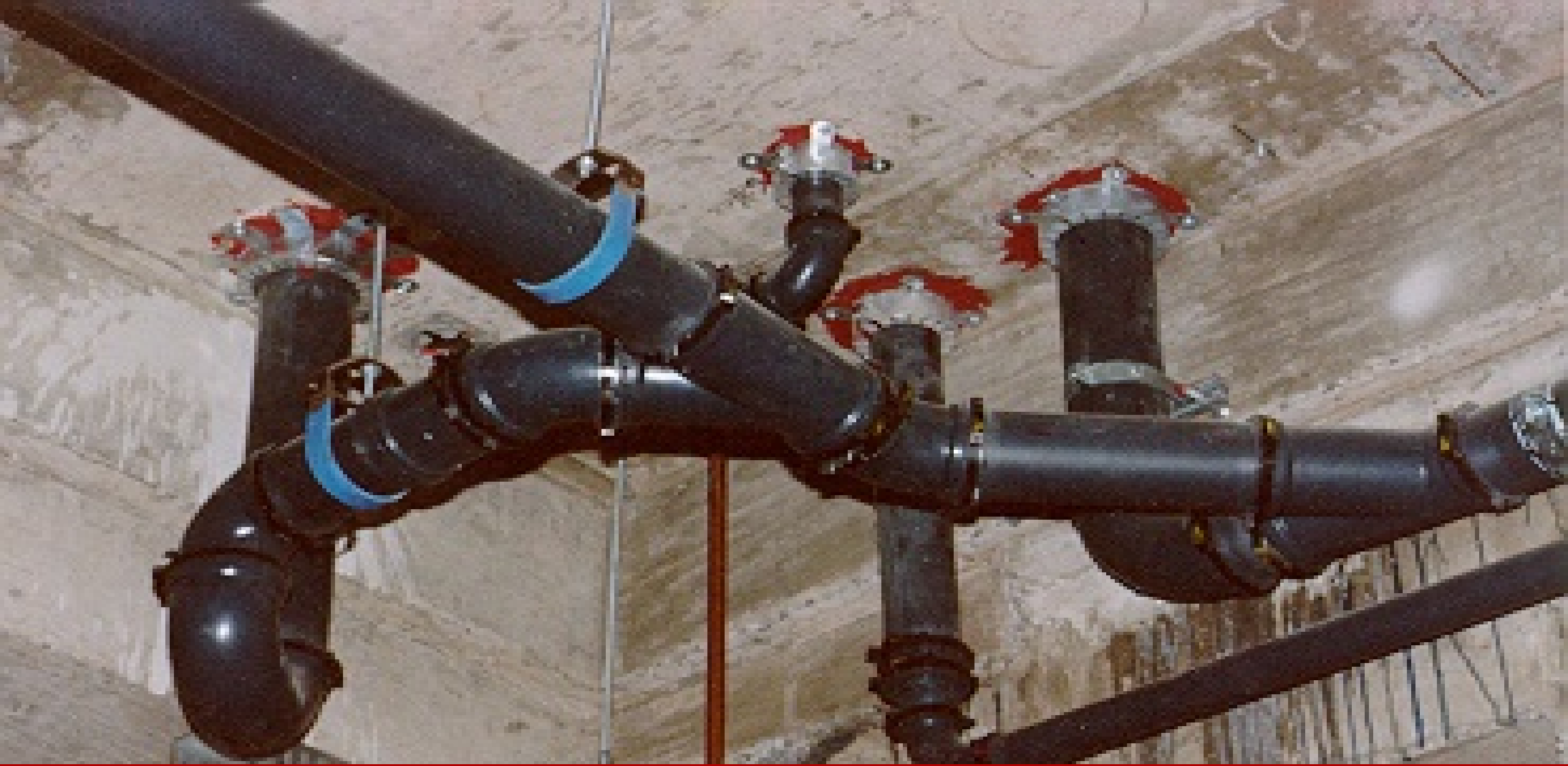
Polypropylene Lab Acid Waste Piping
