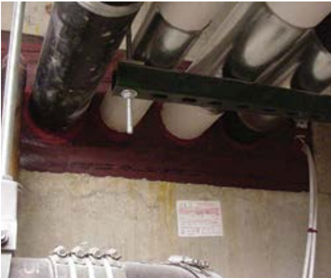
Labels or Tags make system lookup easy. Fire Stop Technologies, Inc. Image
