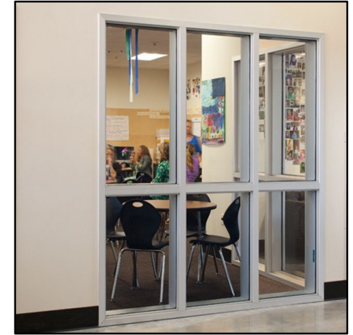
Interior Fire Windows
