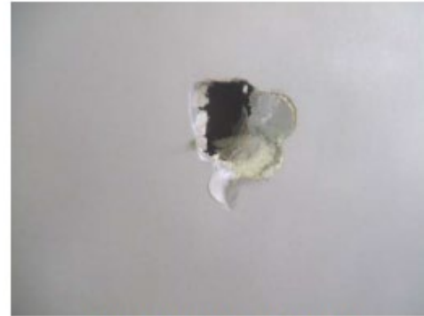
Figure 1: Damaged Gypsum Panel
