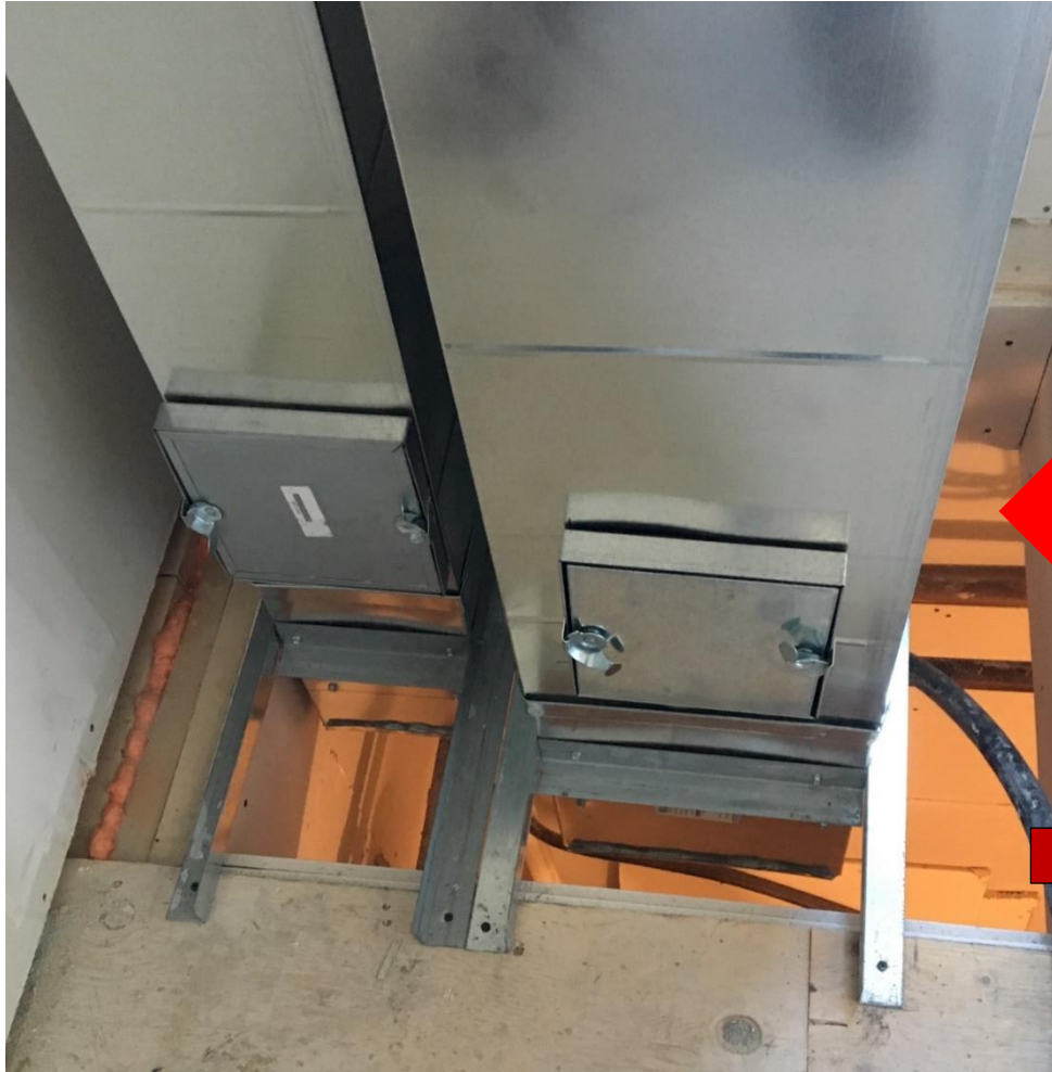
Fire Damper Annular Space?
