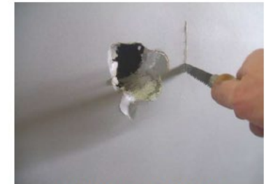
Figure 2: Square Off Damaged Area
