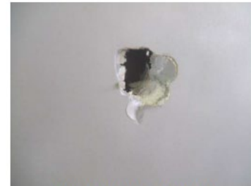
Figure 1: Damaged Gypsum Panel
