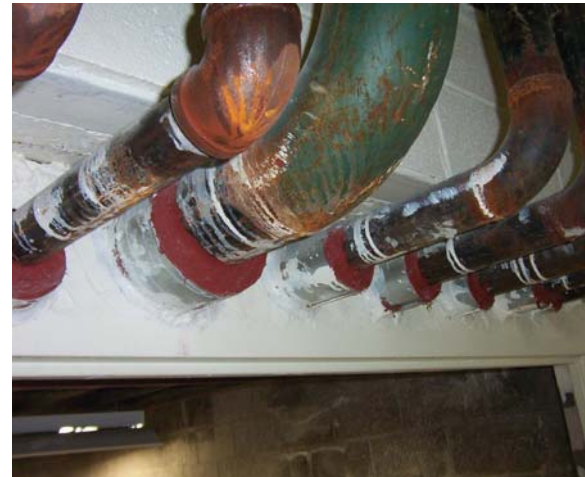
Planning minimizes firestopping costs. (Photo courtesy of Firestop Solutions)
