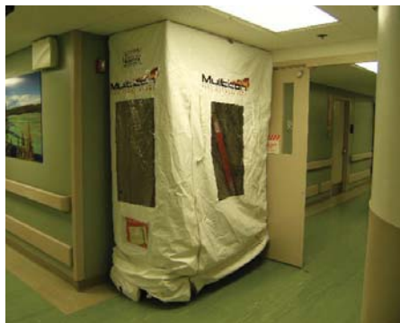
Containment may be required when working above ceilings. (Photo courtesy of Multicon)
