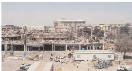
Aftermath of the Santana Row Project in San Jose, Calif. A lower level of concrete and masonry intended for retail space was supporting four stories of light frame construction. This construction would not have met the provisions of international building codes.
