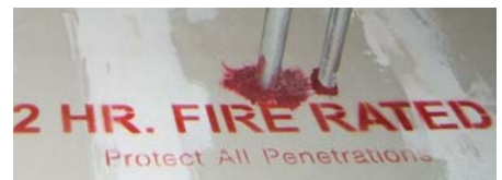
Firestop Systems markings are spelled out in the contractor's quality manual. (Photos courtesy of Multicon Fire Containment)
