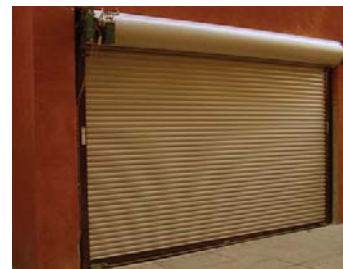
The use of labeled retrofit fire door operators is specifically allowed to replace existing fire door operator, governor and automatic closing systems as long as they are installed in accordance with installation instructions and listings and are acceptable to the Authority Having Jurisdiction.
