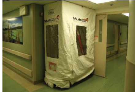
High risk areas need protected work environments.
