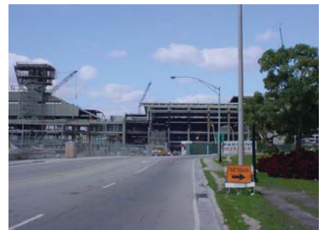
Miami Airport firestopping is a continuous project. (Photo courtesy of Fire Barrier Installations, Inc.)
