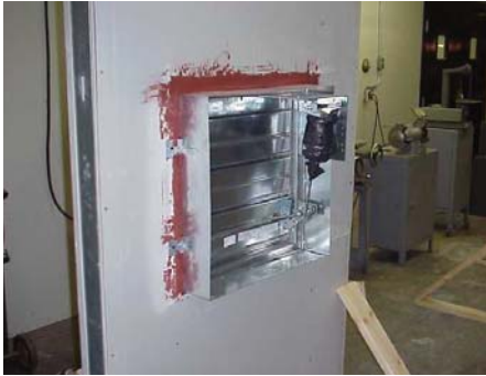
Firestop may be installed, upon damper manufacturer approval. (Photo courtesy of Ruskin)
