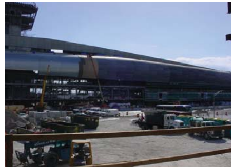
Firestopping around penetrations, head of wall joints and perimeter joints keeps compartmentation working. (Photo courtesy of Fire Barrier Installations, Inc.)
