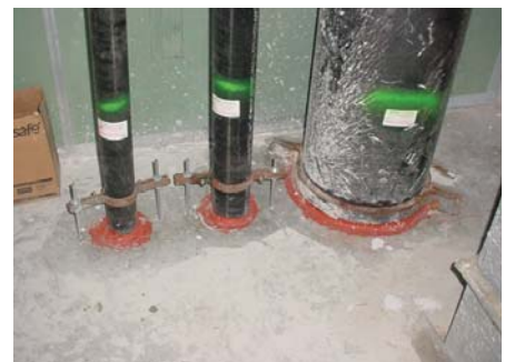
Labels used for identification of firestop system. (Photo courtesy of Fire Barrier Installations, Inc.)
