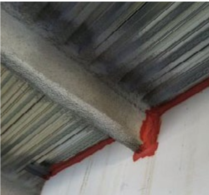
HW assembly, metal deck flutes running parallel to the wall. Fire Stop Technologies Photo
