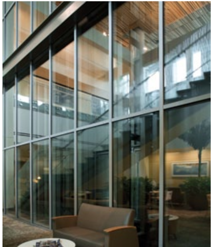
A fire-resistance-rated glass curtain wall creates a light, open lobby. TGP Photo
