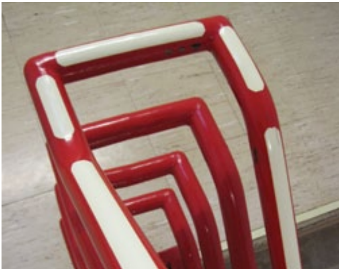
Top surface of handrail with gaps up to 4-inches. American Permalite Photo
