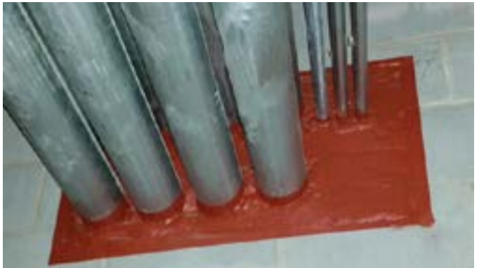
New breaches need repair to maintain barrier fire-resistance-ratings and smoke-resistant properties. Fire dampers, fire doors, fire-rated glazing, and blank holes have requirements for maintenance in the International Fire Code, NFPA 1, NFPA 101, NFPA 80, and more. Even wall patches need to be fire-resistance-rated. The top image shows an improperly firestopped penetration. The bottom image appears to show a proper firestop installation, though it would have to be verified against the installed tested and listed system specs to confirm proper installation. Affinity Firestop Photos
