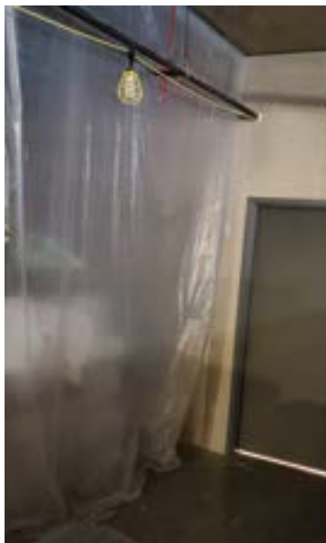
Common deficiencies include wires not permitted to be attached to sprinkler piping and excessive door gap allowing particulate to leave the construction area. Credit: CCI
