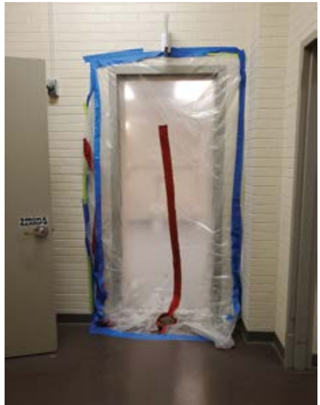
Typical plastic barrier installed for infection control purposes not properly secured and not closed after entry by contractor staff. Credit: CCI Photo.
