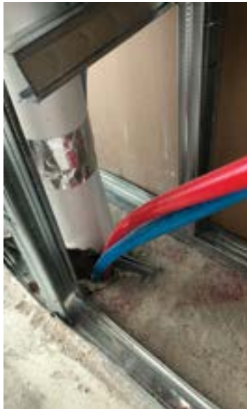
Breaches in fire- and smoke-resistant assemblies are to be protected, continuously. Maintaining protection is mandated by fire codes. J. Sharpe Photos
