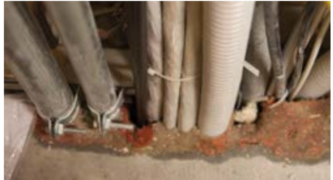
Required compartmentation breached by cabling, pipes, not protected properly. K. Heckler Photo
