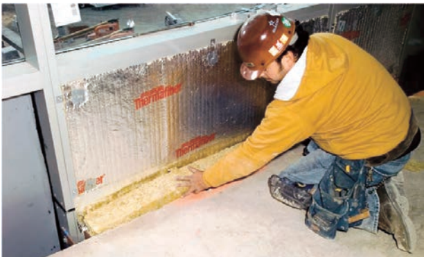
Firestop Containment Workers install systems and engineering judgments. Thermafiber, an Owens Corning Company Photo
