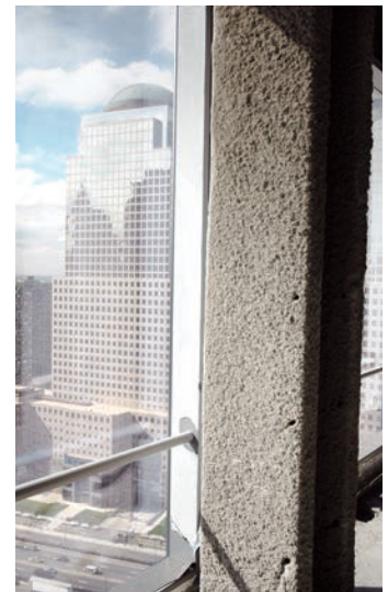
Steel columns with SFRM Fireproofing protection. Photo of Grace Monokote MK-10HB. Grace Photo.
