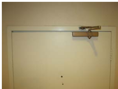
Excess clearance around a fire door will affect smoke infiltration, as well as the performance of the assembly during a fire. Allegion Photo
