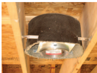
Recessed light with fire rated light cover. Tenmat Photo
