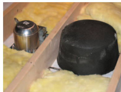
Unprotected recessed light next to properly fire rated light. Tenmat Photo
