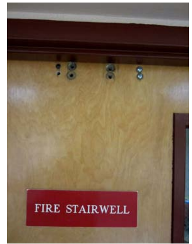
When the door closer on this fire door was replaced, the resulting holes should have been filled with steel fasteners or a material that is approved for this use. Allegion Photo
