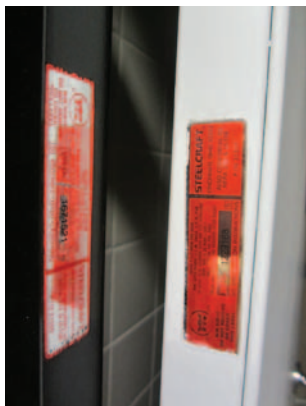
Labels located on the door edge and frame rabbet include important information about the fire door assembly and must remain legible. Allegion Photo
