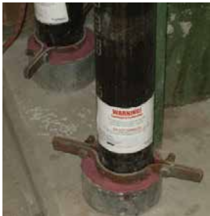
Firestop Products installed in a sleeve to a FM, UL or other listing laboratory detail becomes a SYSTEM. Note identification label for system. FCIA Photo.
