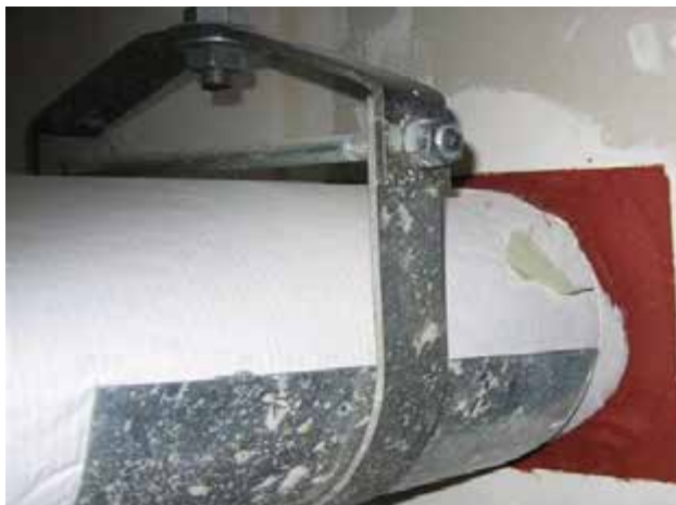
Pipe properly firestopped through a penetration. Firestop Solutions, Inc. photo
