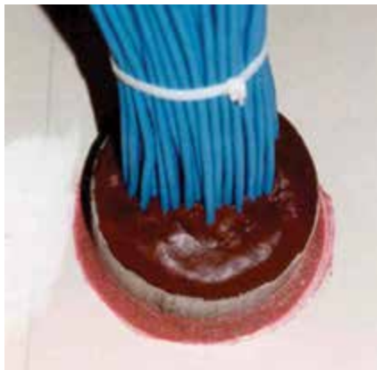
Multiple cables firestopped. Firestop Solutions, Inc. photo
