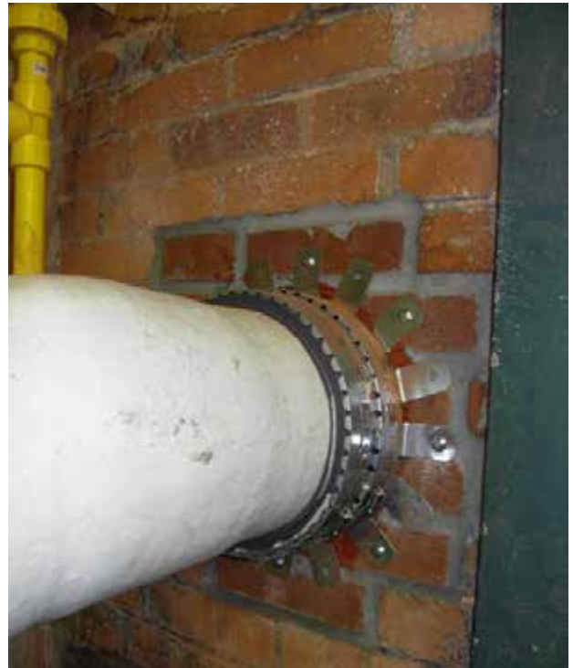
Pipe firestopped through a fire resistance rated brick masonry wall. Firestop Solutions, Inc. photo
