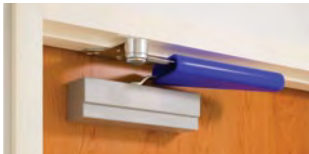
The 2018 model code language prohibits modifications to panic hardware, fire door hardware, and door closers. Hardware used on fire doors must be listed for that purpose. Allegion photo
