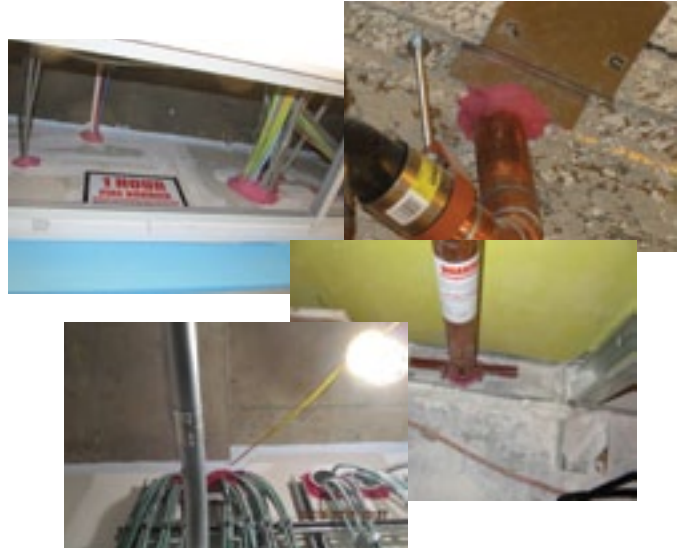
Penetrating items through breaches in Fire Barriers. Photos: Gleeson Powers
