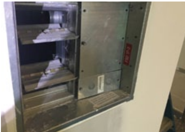
Example of a Fire/Smoke Damper SGH photo
