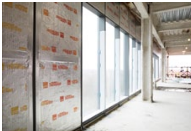
Building codes require a barrier to prevent the spread of fire from the interior joint where a void exists between the fire-rated horizontal assembly perimeter joint and the exterior non-rated curtain-wall. Owens Corning/Thermafiber photo.
