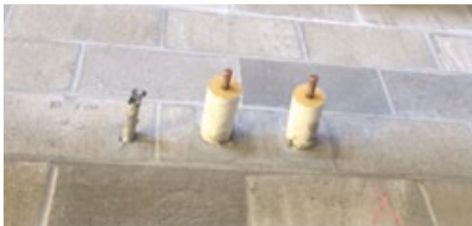
Small annular spaces mean it is difficult to get full thickness of the block or enough mortar to meet the fire-resistance-rating. Note that insulated penetrating items are not allowed to have mortar installed according to the International Building Code. Cement mortar is not compatible with copper piping. Fire Stop Technologies Photo
