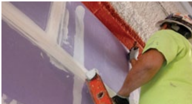
Firestop Inspection Agencies need to supply inspectors with ladders. Firestop Southwest Photo.
