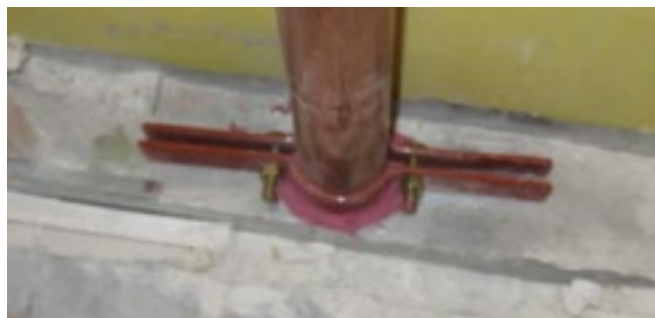
Firestopping looks easy. Annular space sizes, backing/damming depth, firestop sealant application under pipe supports, correct firestop sealant thickness, and then, documentation of the UL System, (F-A-1068) is key to success. Gleeson Powers Photo
