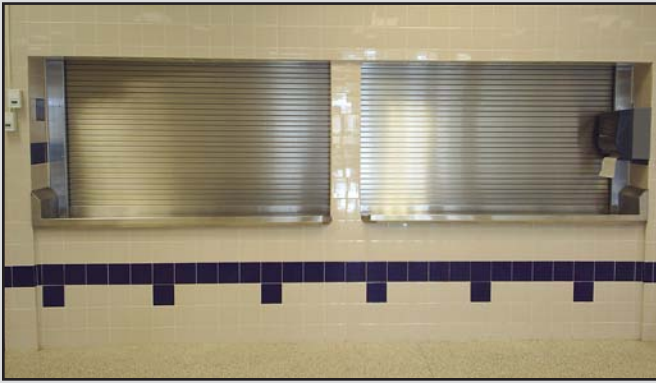
Rolling Fire Doors can be single, or side by side separated by fire resistance rated assemblies. Cornell Photo
