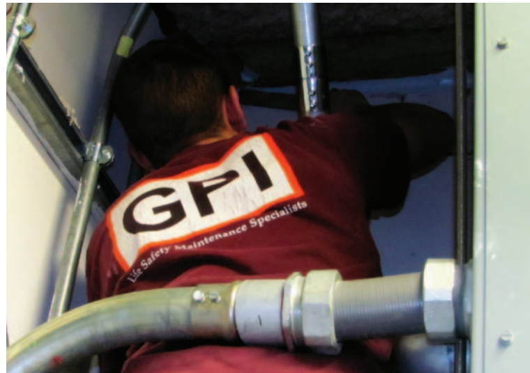
Barrier management means reviewing conditions above ceilings to get to fire-resistance rated construction. Gleason Powers Photo
