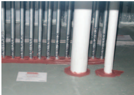
Firestopping can be labeled by contractors who understand the zero tolerance firestop systems protocol. PPMI photo
