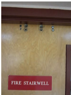
Holes Left in Door and Missing Fasteners. Ingersoll-Rand Photo.
