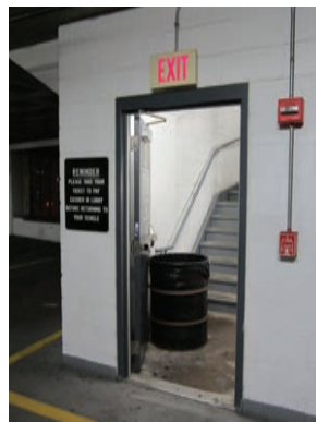
Stairwell Door Propped Open. Ingersoll-Rand Photo.
