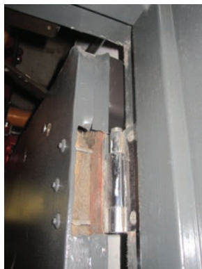
Missing Hinge Reinforcement. Ingersoll-Rand Photo.
