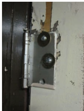
Hinge with Wrong and Missing Fasteners. Ingersoll-Rand Photo.
