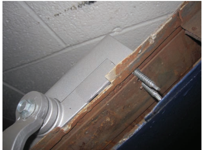
Missing Top Channel. Ingersoll-Rand Photo.
