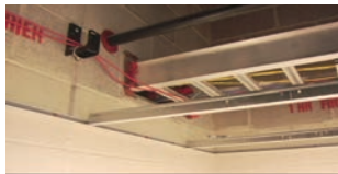
Smoke barriers protect patients from fire and resist smoke. FCIA Photo.
