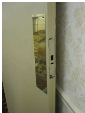
Missing Latch. Ingersoll-Rand Photo.
