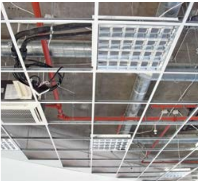
The plenum area hosts pipes, as well as networks and ducts of varying sizes and configurations. iStock.com/Andaleks3 photo
