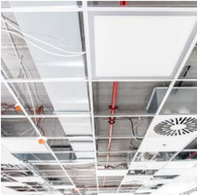
As plenum areas can be challenging to access, it is important that materials such as insulation jacketing stay sealed. Lukassek/Shutterstock.com photo
