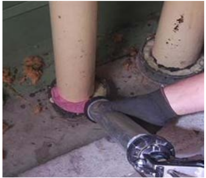
In this case, the firestop product is installed above the mineral wool at the top of the sleeve. The tested and listed system sometimes states to install at the plane of the floor. Firestop Contractors pay attention to systems and know to look for this positioning. FCIA Photo
