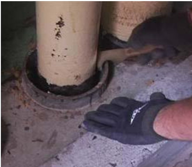
In UL Firestop System C-AJ-1353, for existing buildings, the surfaces must be cleaned free of dirt, debris, paint. FCIA Photo
