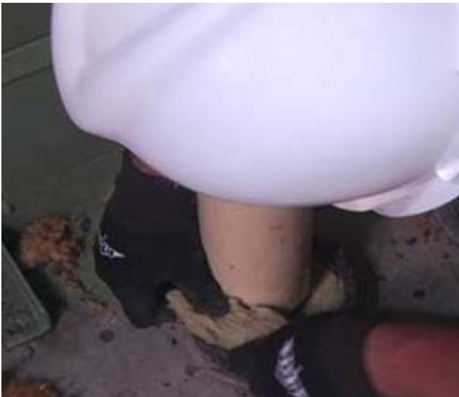
Firestop Containment Workers install backing/damming materials such as mineral wool to the C-AJ-1353 system specified thickness, depth and density. FCIA Photo
