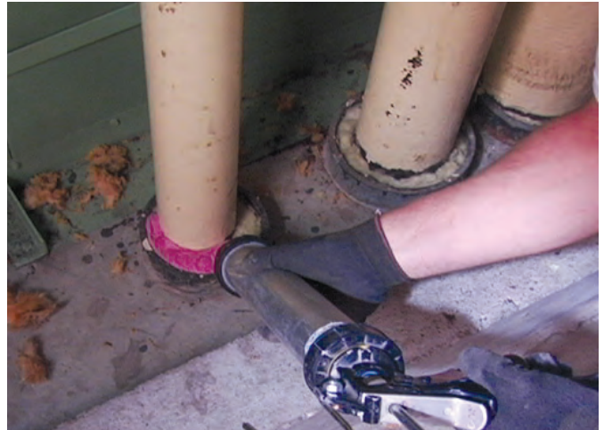
Intumescent firestop sealant fill, void or cavity materials installed over backing/damming. FCIA Photo
