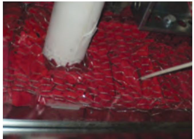
Firestop bags used as fill, void or cavity material. FCIA Photo
