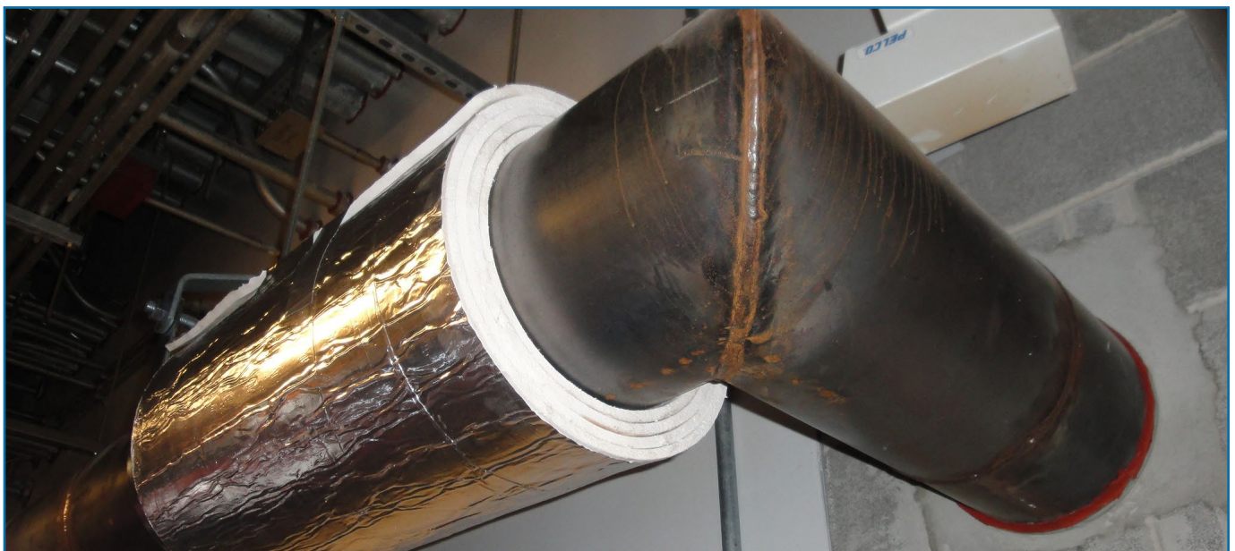
Fire-resistant pipe-protection system during installation on horizontal offset fuel pipe. Photo courtesy of 3M Fire Protection Products
