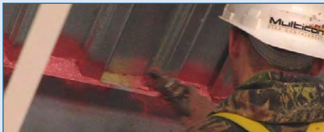
What if a penetrating item went into the Head of wall? System violation. FCIA Photo
