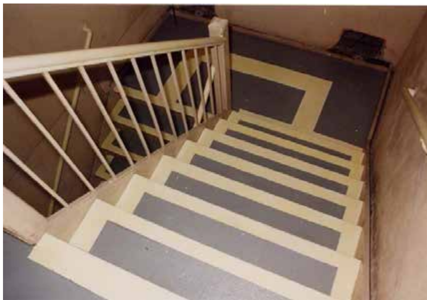
WTC NYC Photoluminescent Step, Landing and Handrail Markings 1994. (Photo: Copyright PERMALIGHT®.)
