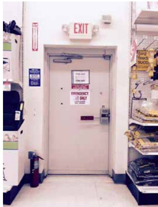
Figure 3: Confusing Signage on Emergency Exit Door (Photo courtesy of Scott Tobias.)
