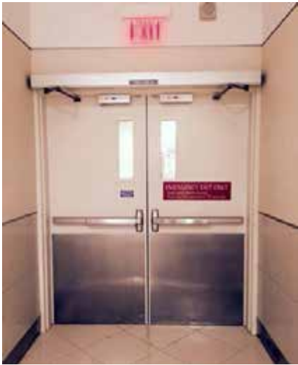
Figure 2: Clearly marked and lit Fire Door (Photo courtesy of Scott Tobias.)
