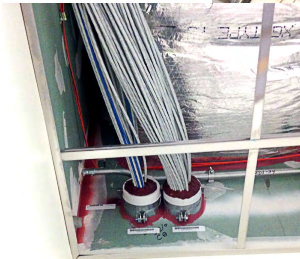
Insulated HVAC duct firestopped using SpecSeal® Triple S Sealant (above). Conduit sleeves shown above the ceiling grid penetrating a 1-hour fire-rated barrier firestopped with SpecSeal® SSP Putty with sleeve around the cables and SpecSeal® Triple S Sealant around the sleeve (below). STI Photo
