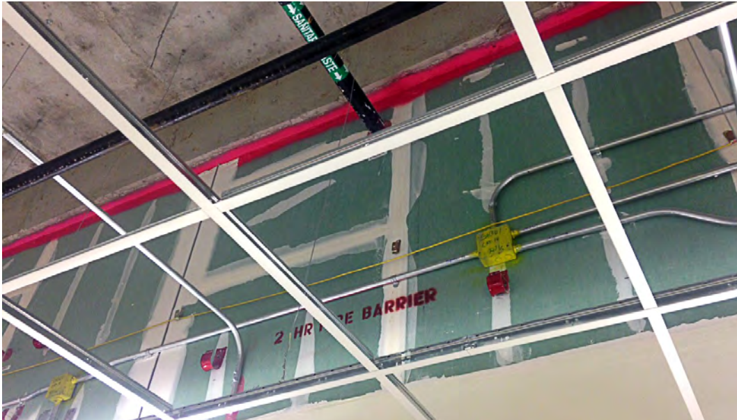
Head of wall joint shown above the ceiling grid packed with mineral wool and encapsulated with SpecSeal® AS200 Firestop Spray applied on both sides of wall used to preserve the 2-hour fire rating. STI Photo
