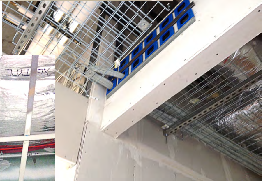
Twelve individual EZ-Path® Smoke & Acoustical Pathway Modules (Catalog No. NEZ33) with field fabricated mounting plates penetrating a non-rated partition. STI Photo
