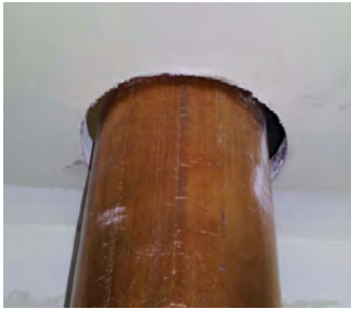
Copper Medical Gas Lines
