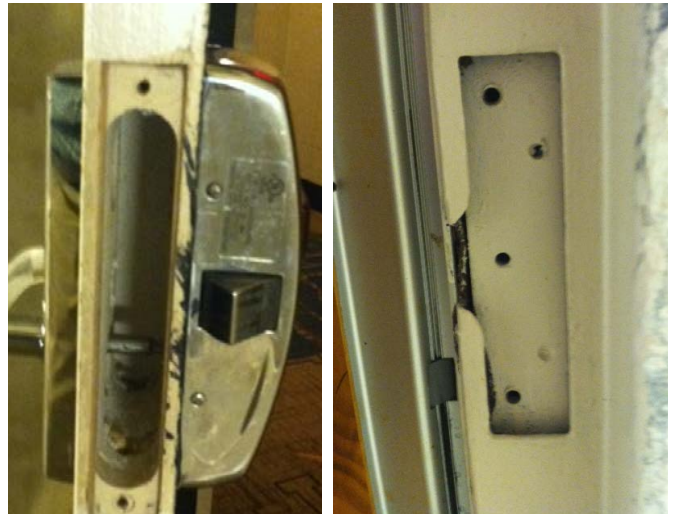
Non-compliant door field modification
