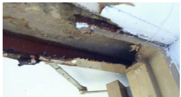
Rusted through door frame
