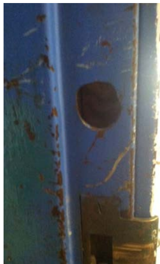
Holes in door frame jamb
