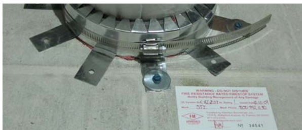
Labeling identifies the firestop system reducing inspection costs. FCIA Photo
