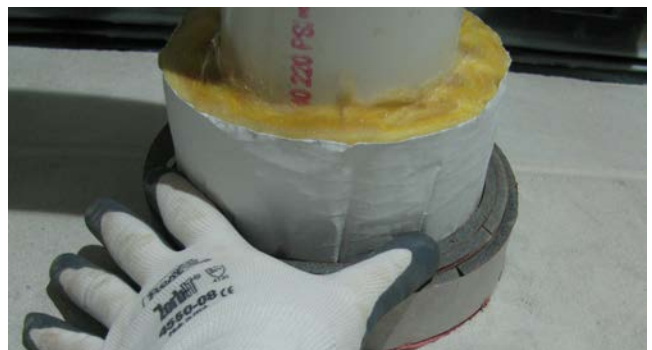
Firestop installations can be viewed by special inspection personnel as being installed or destructively tested. FCIA Photo
