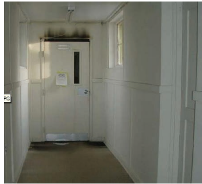
Fire doors protect people and property. Foundation for Life Safety and Security Photo
