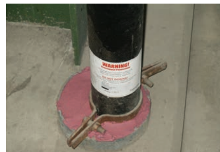
Floor through penetration firestop systems are generally easy to inspect. PPMI Firestop Photo
