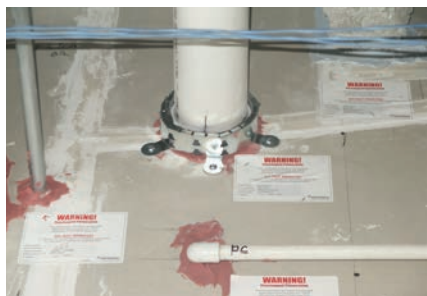
When firestopping is labeled, inspection is much more efficient. PPMI Firestop Photo
