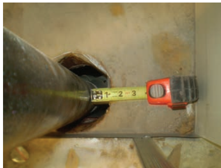
Measuring annular space size for compliance to listed system depth. Hamilton-Benchmark Photo
