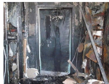
Damage kept in the compartment of origin by fire resistance rated wall and fire door and its glazing protecting the opening from fire spread. Fire Doors that were closed, like this, worked in Chicago. Foundation for Life Safety and Security Photo
