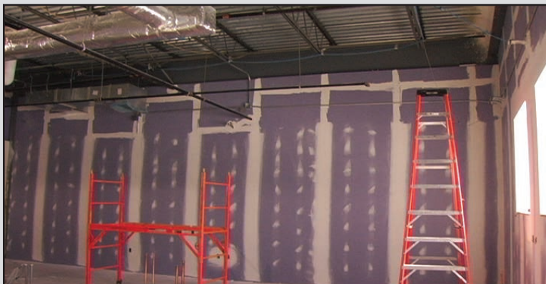
Fire resistance rated construction protects people in buildings. FCIA Photo
