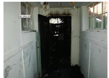
Note the smoke around the door and frame interface at the top. Foundation for Life Safety and Security Photo
