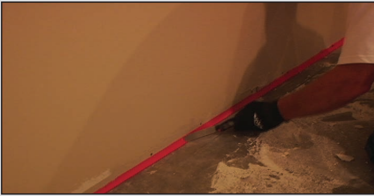
Firestopping is installed at the top and bottom of walls for continuity of the fire resistance rating. FCIA Photo
