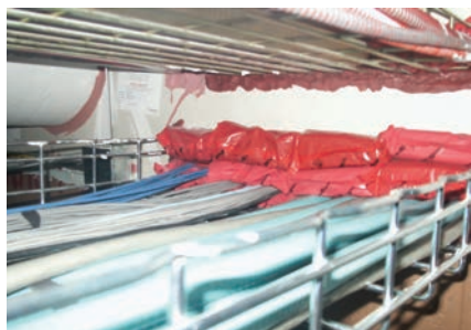
Firestopping is often harder to get to than inspect. PPMI Firestop Photo
