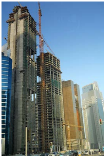
Throughout the world, safety is designed and engineered into buildings. FCIA Photo
