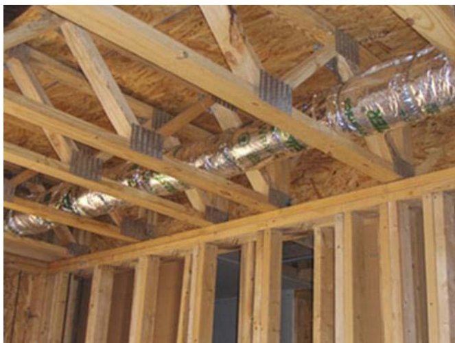
Figure 1 – Ventilation in space above ceiling, below floor. Thermal Ceramics Photo.
