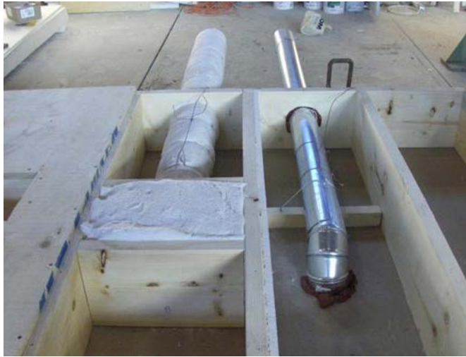
Duct B Duct A Figure 3 – Thermal Ceramics Photo
