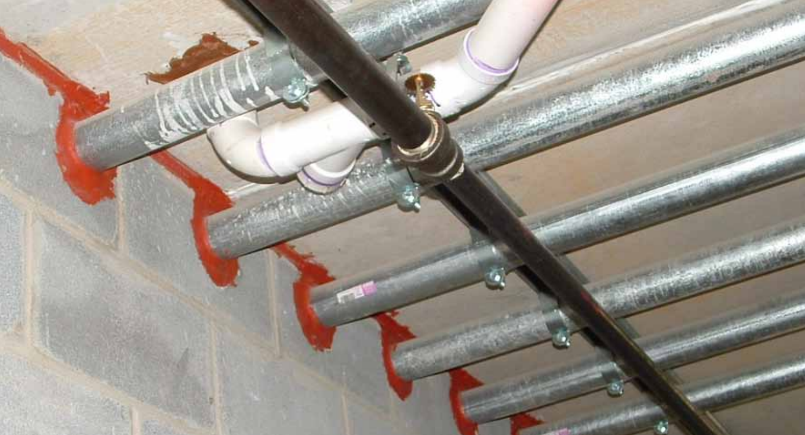
Walltop firestop systems with pipes need a system that allows pipes, and not just a joint. Premier Firestop Photo
