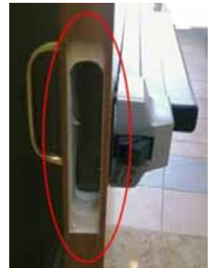
Parts missing, inoperable pull side. DHI photo
