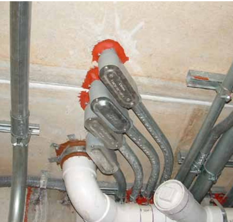
Firestop / Containment Workers and Firestopping Special Inspection Agencies understand the limitations of system designs. Premier Firestop Photo
