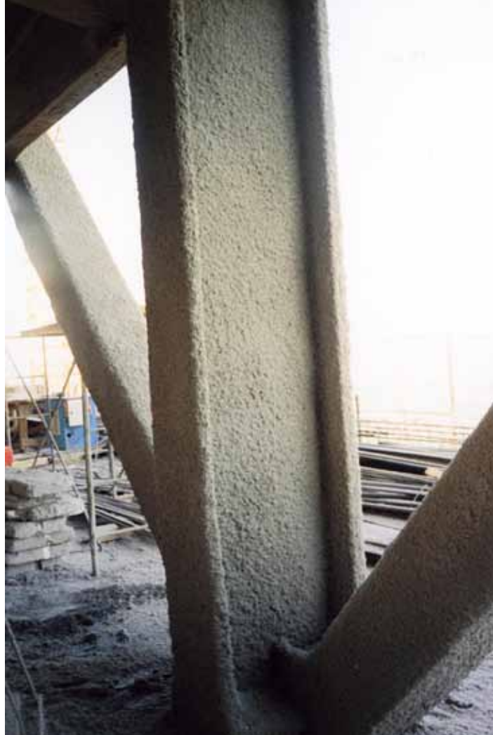
Above. Dry spray SFRM applied to steel columns and bracing members. ISOLATEK photo
