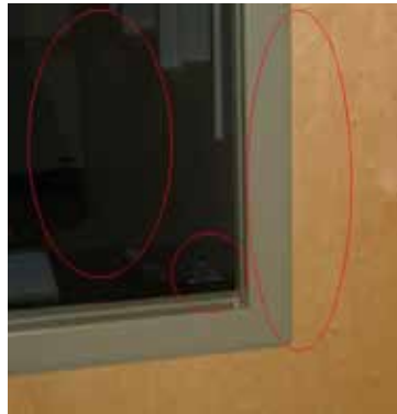
Check glass label, frame, glazing per code requirements. DHI Photo
