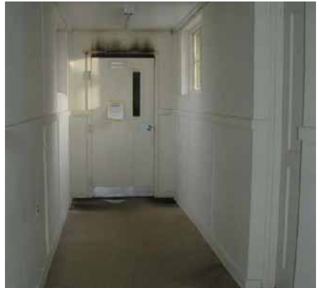
Fire door acting as intended. Note smoke stains from fire. DHI Photo
