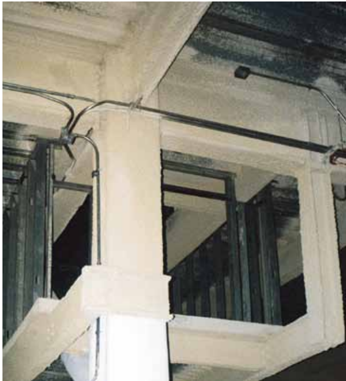
Above. Wet Spray SFRM applied to steel columns, beams and bracing members. ISOLATEK photo
