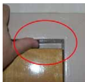
Examine gap around frame. DHI Photo
