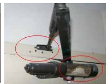
Holes in frame, closer leaking. DHI Photo
