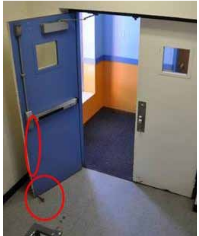
Wood stop, bottom rod removed. DHI Photo
