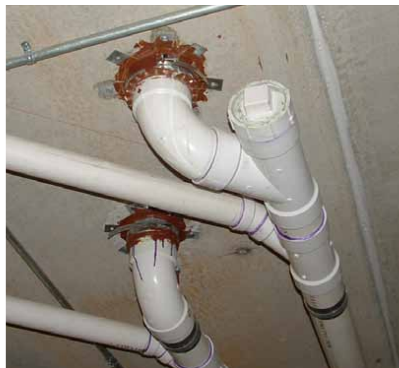
Fire resistance rated floors with plastic drain pipes in parking garages located under multi-family unit residences are protected with wrap strips and collars or plastic pipe devices. Tabs must be folded 90 degrees to conform to the system. Premier Firestop Photo
