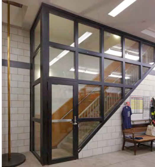
Stairwells with visible features and fire rated. - Pilkington Photo
