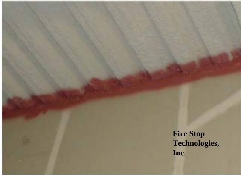
Fire Stop Technologies, Inc.
